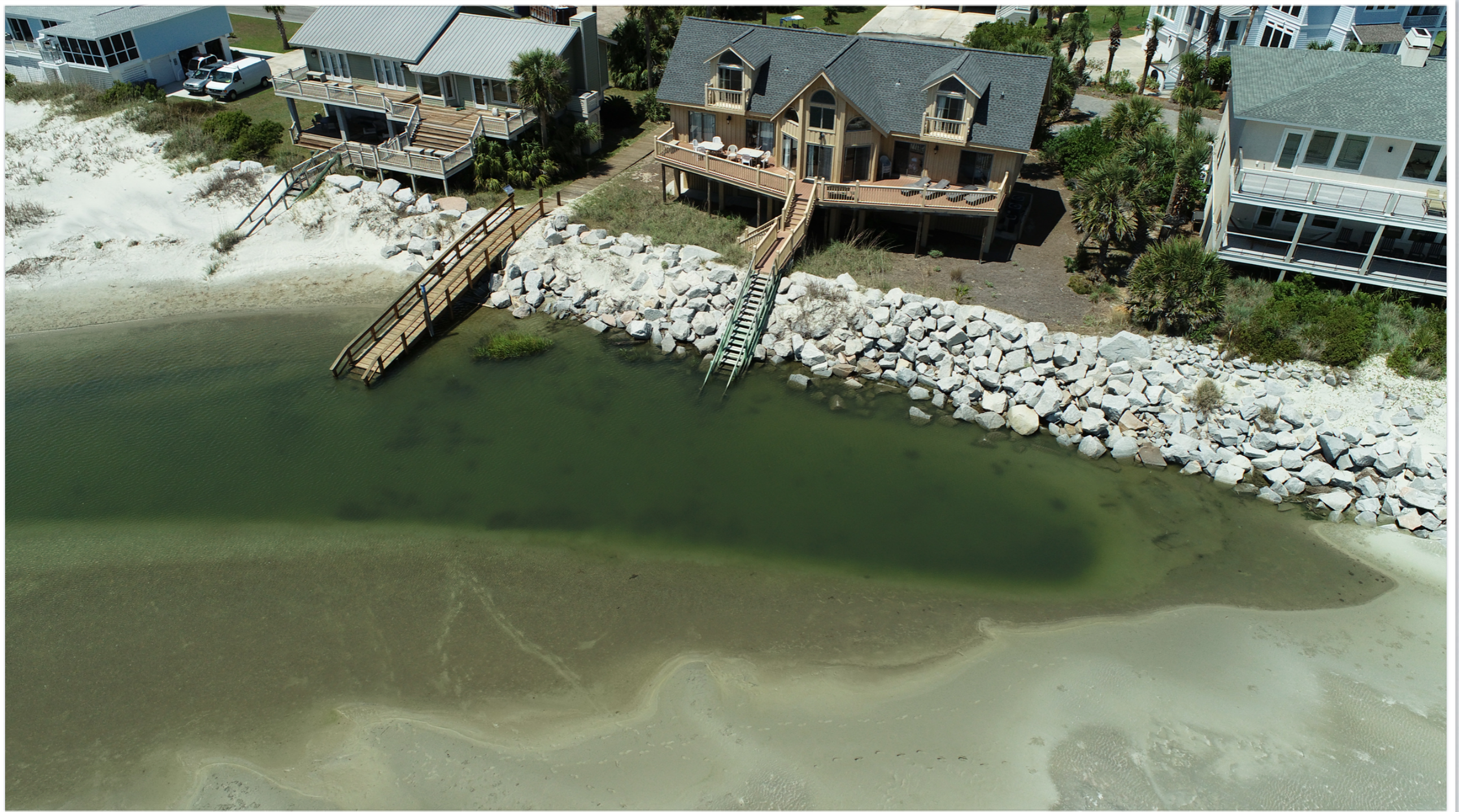
Access #1b - Overall view of access #1b as it sits in relation to the tide pool that has formed at the end of it. It is currently inaccessible.
