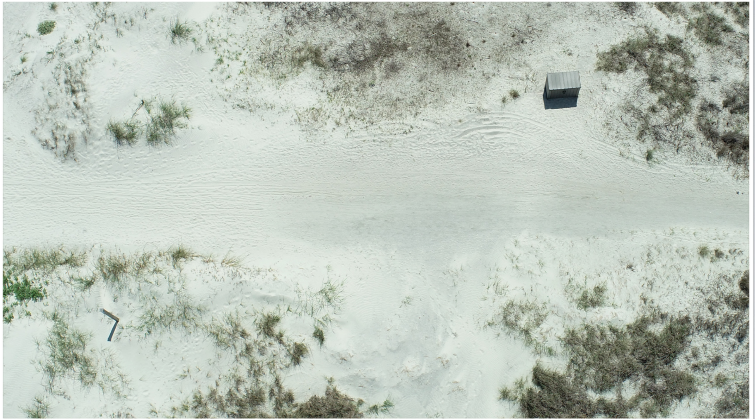
Access #15. Closeup view. People are walking/driving along the side of the geo-webbing for the last 100 feet or so. Less foot traffic on the webbing allows it to be taken over by encroaching sand dunes.
