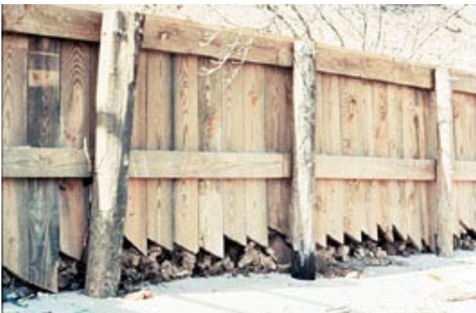
Figure 8. Loss of backfill and eventual bulkhead failure is the result of sheeting not driven to sufficient depth.
