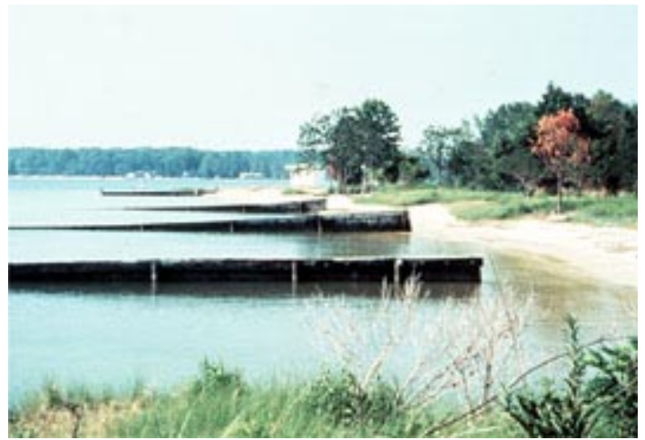
Figure 57. Groin field flanked by erosion.
