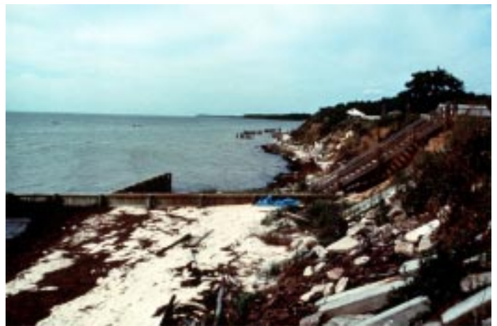
Figure 53. Sand accumulated on updrift side of groin.
