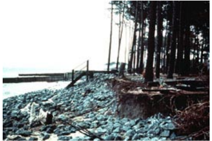
Figure 18. Revetment in Figure 17 failed after a storm.
