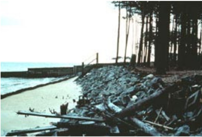
Figure 17. Underdesigned revetment before storm.
