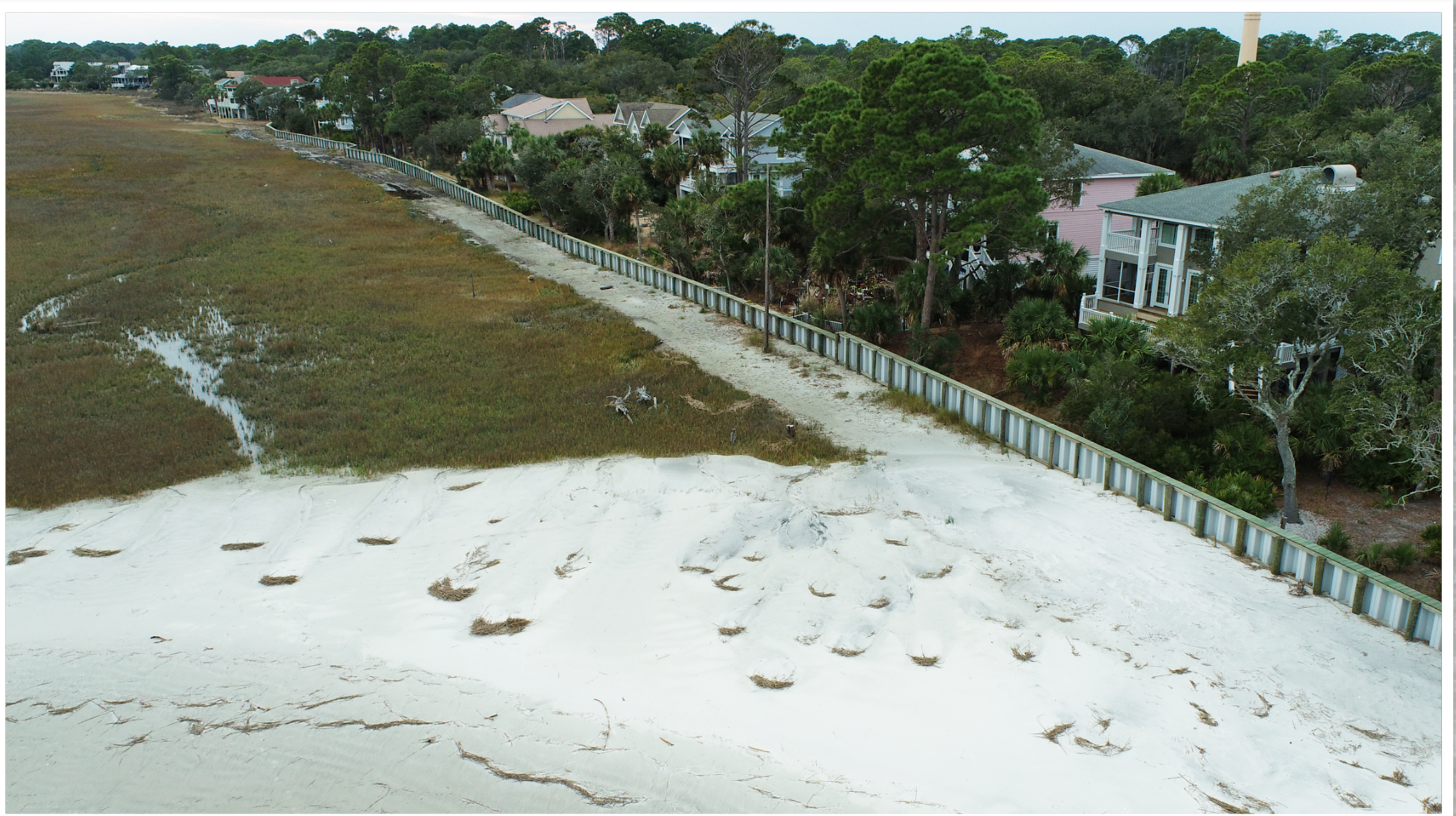
Another view, taken on January 21, 2022 , shows the sea wall extends down Cardinal Crest Lane, but does not go the full length of the marsh. Eventually it will have to if the marsh continues to deteriorate or any opening will become a weak link in the chain.
