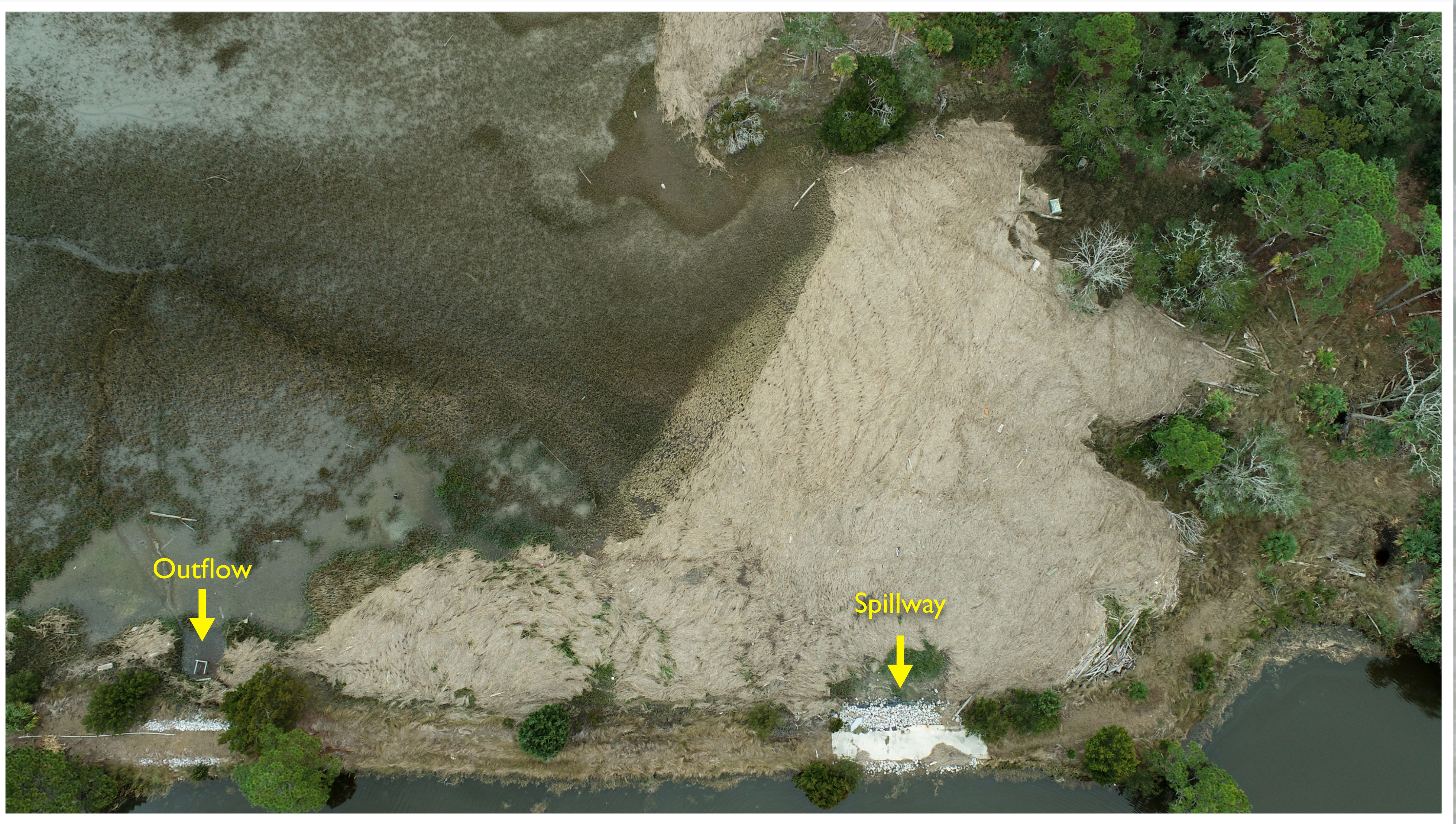
The amount of wrack piled up against the spillway and surrounding area could ultimately act like a dam in front of the spillway causing flooding in other areas during higher than normal tide events. A large amount of wrack gets pushed into the interior lakes, which causes them to become shallower, effecting the amount of runoff drainage that can occur within the interior of the island.
