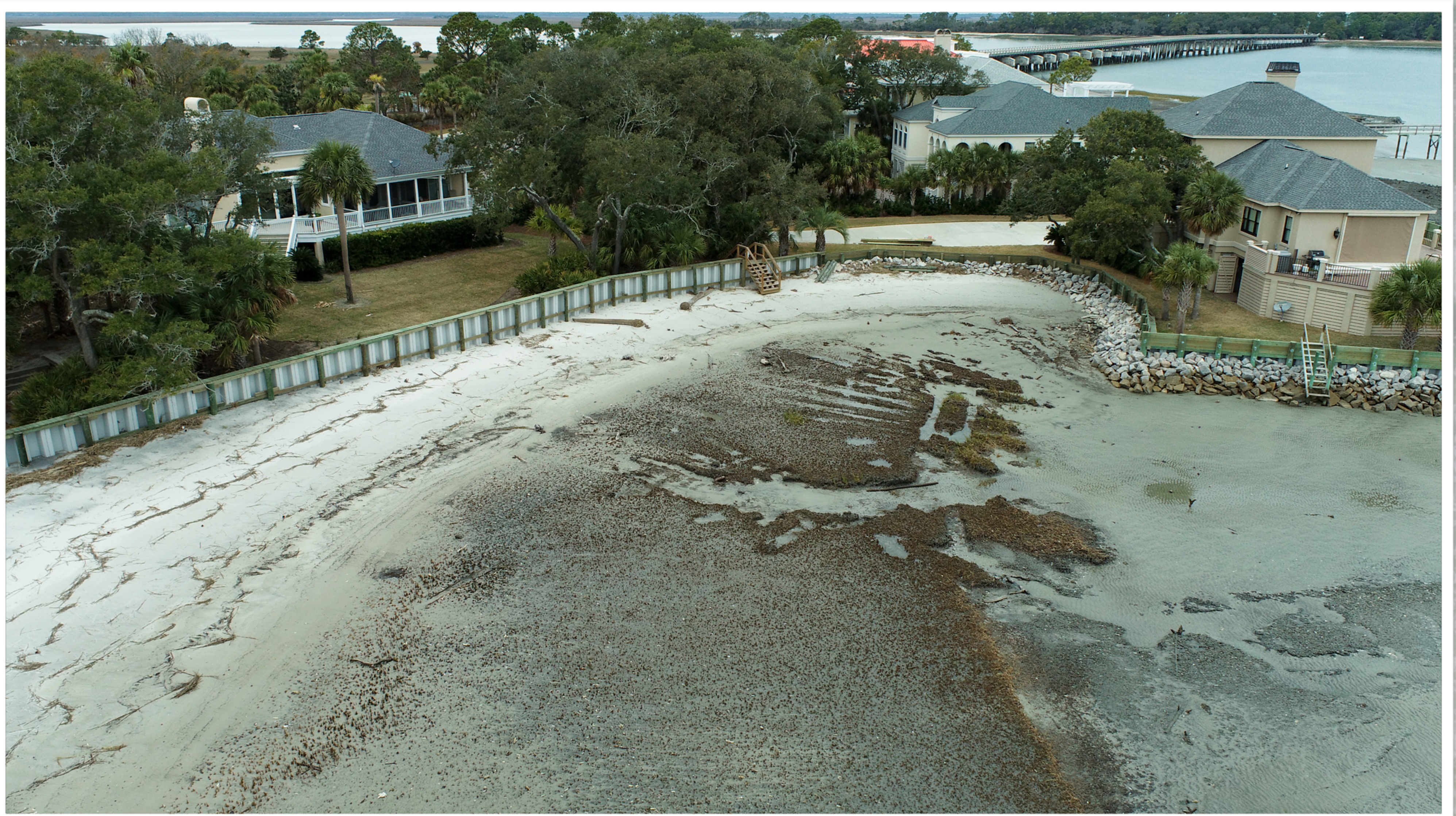
Another view of the eroded area, taken on January 21, 2022 . The sea wall in this corner is the main barrier that prevents sea water from flooding the River Club neighborhood and Tarpon Boulevard during king tides or storm events.
