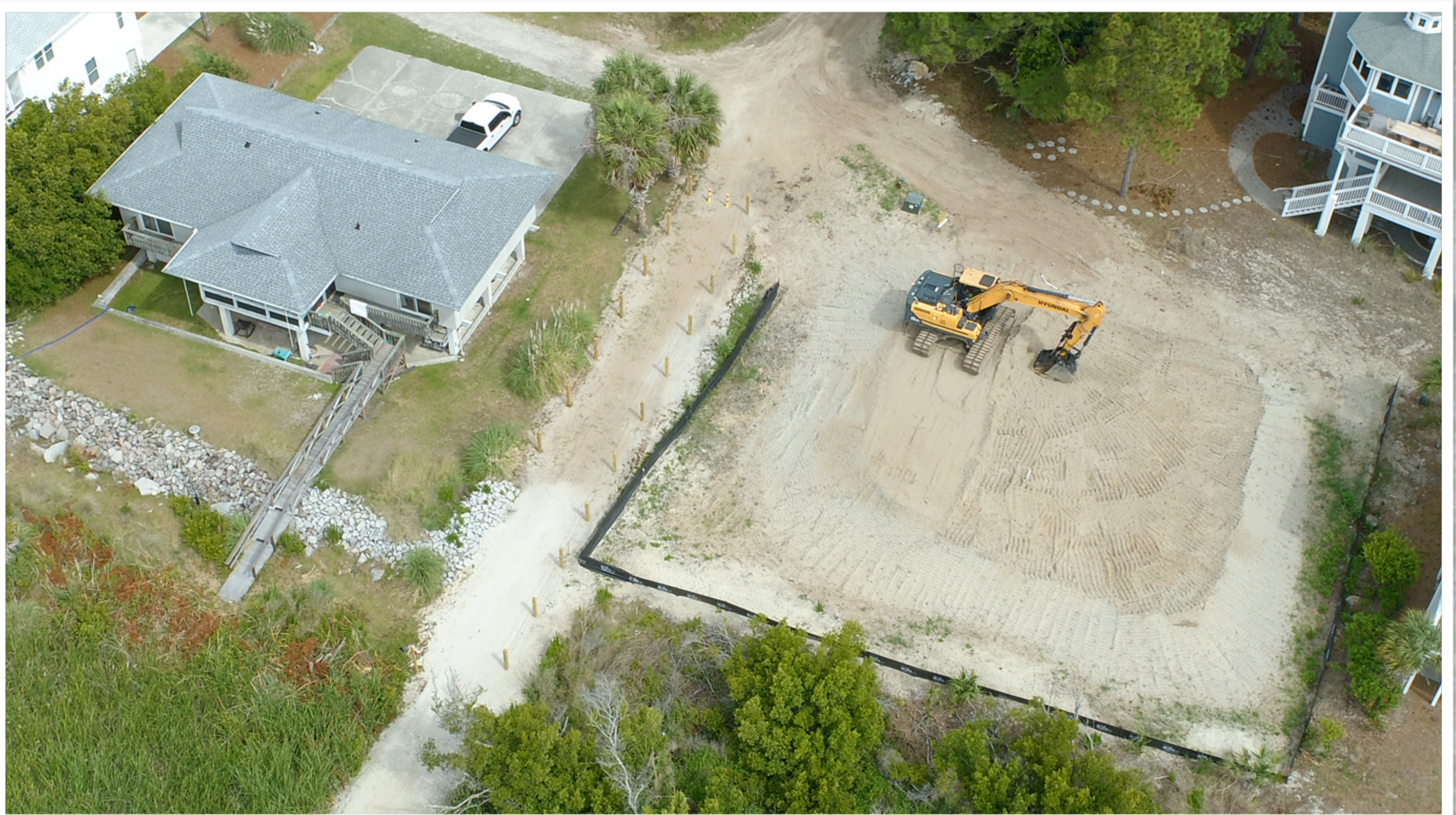
Detail of access #4 - entrance - Posts and bollards in place. Ropes to be added connecting each post preventing the bypassing of the bollards by unauthorized vehicles.
