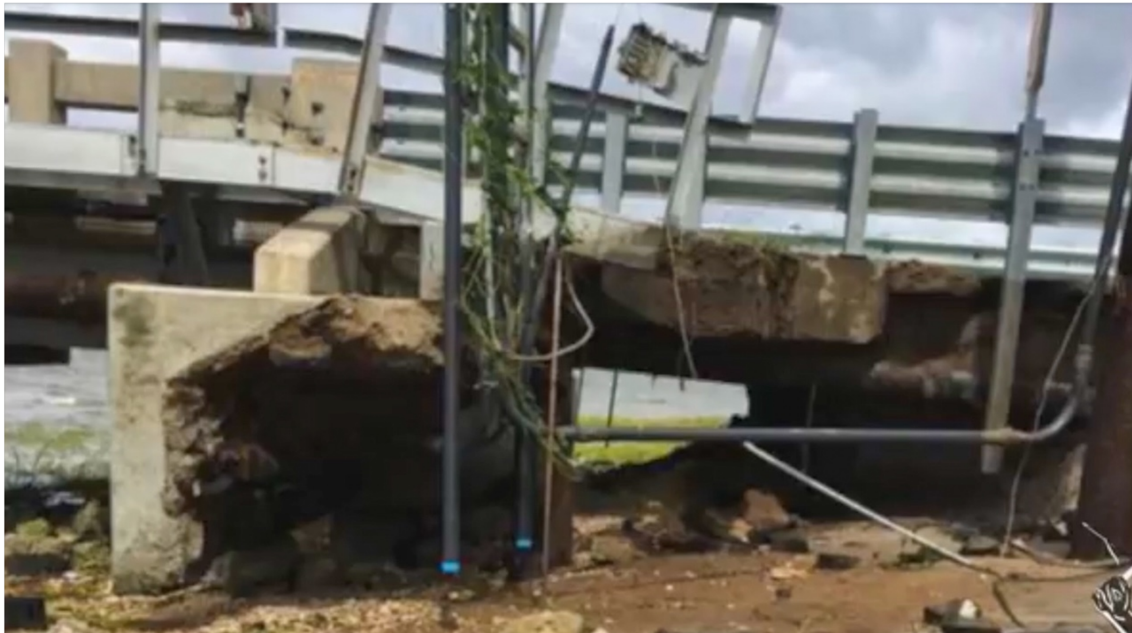
Harbor River bridge hurricane Matthew
