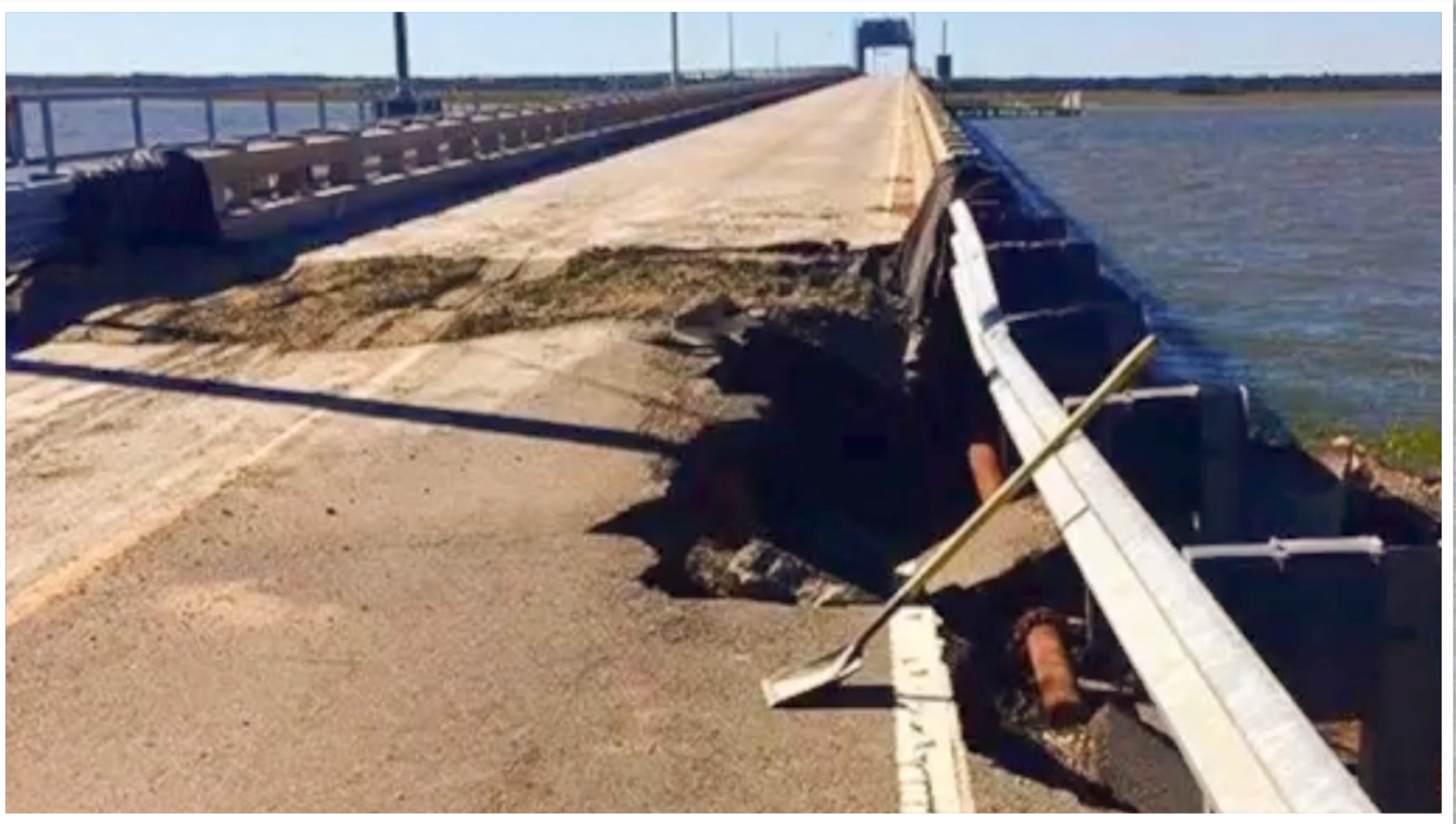
Harbor River bridge hurricane Matthew
